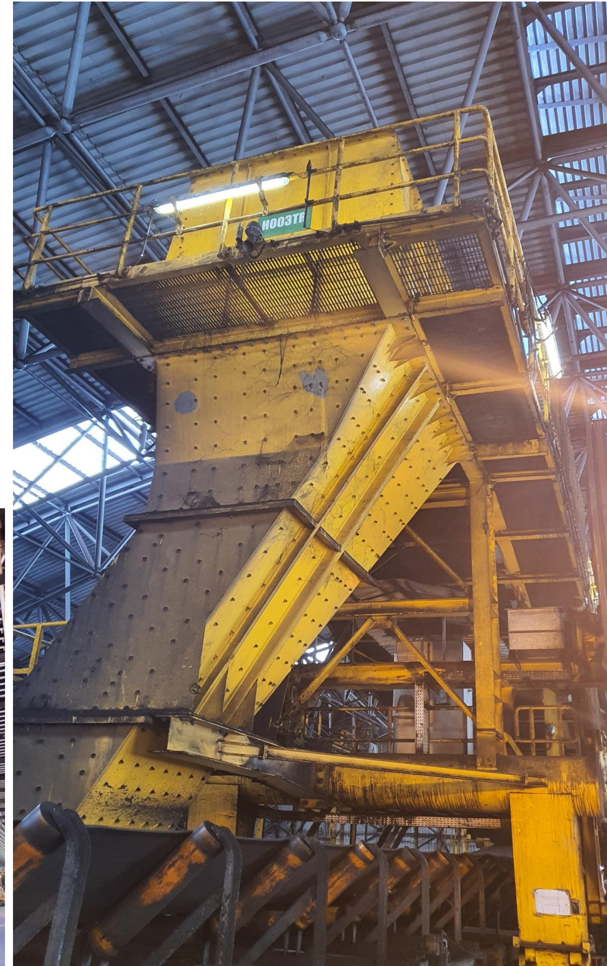
2. Tripper Car Conveyor
